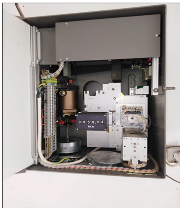
Fig. 4 Water level sensor fixed in the Qaraaoun Reservoir
